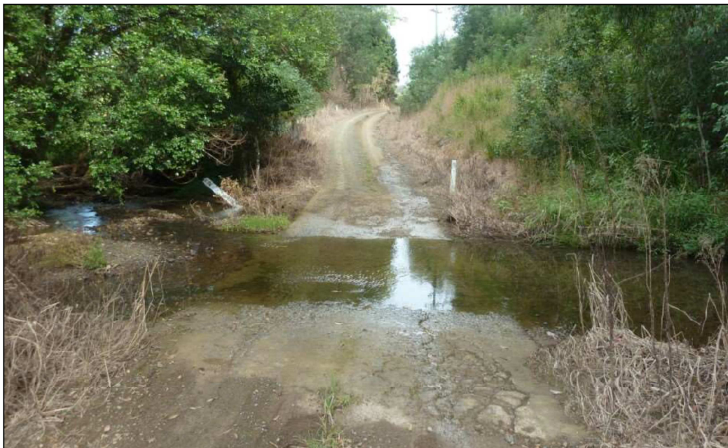
Example of a water crossing requiring management in the Hunter region. (photo: HCCREMS)
